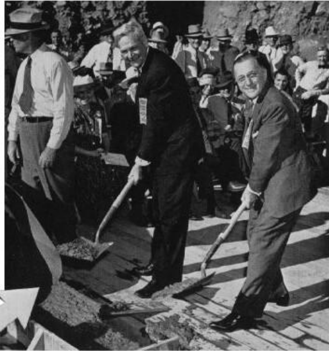
● Left, General Manager Weymouth. Center, the completion ceremony. Right, Chairman Whitsett and Director Rossetti place the last concrete in the main aqueduct. ●
